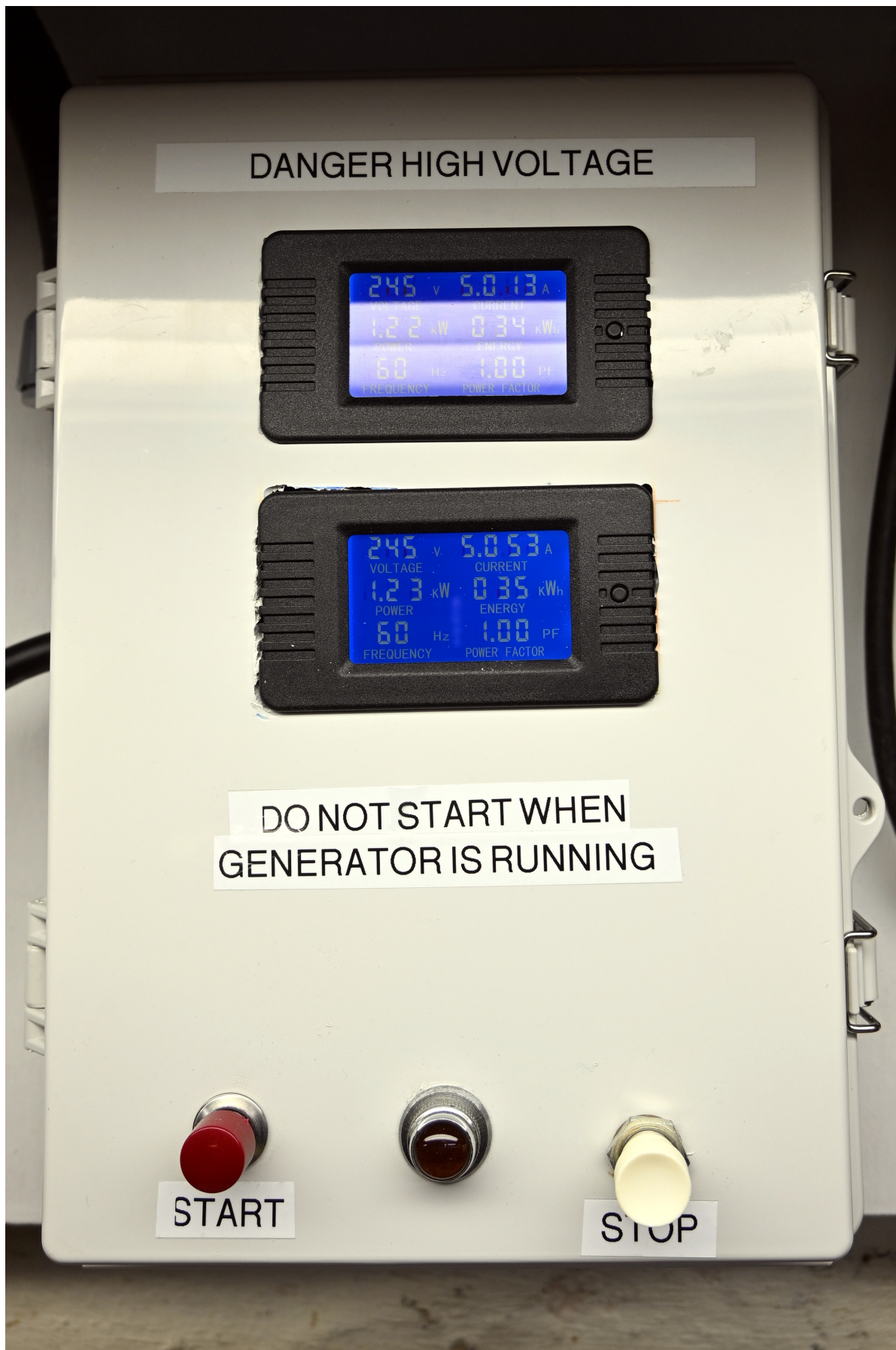
Control box located in the basement. This will disconnect the panels in the rare event of a power failure protecting my natural gas 20KW generator.
