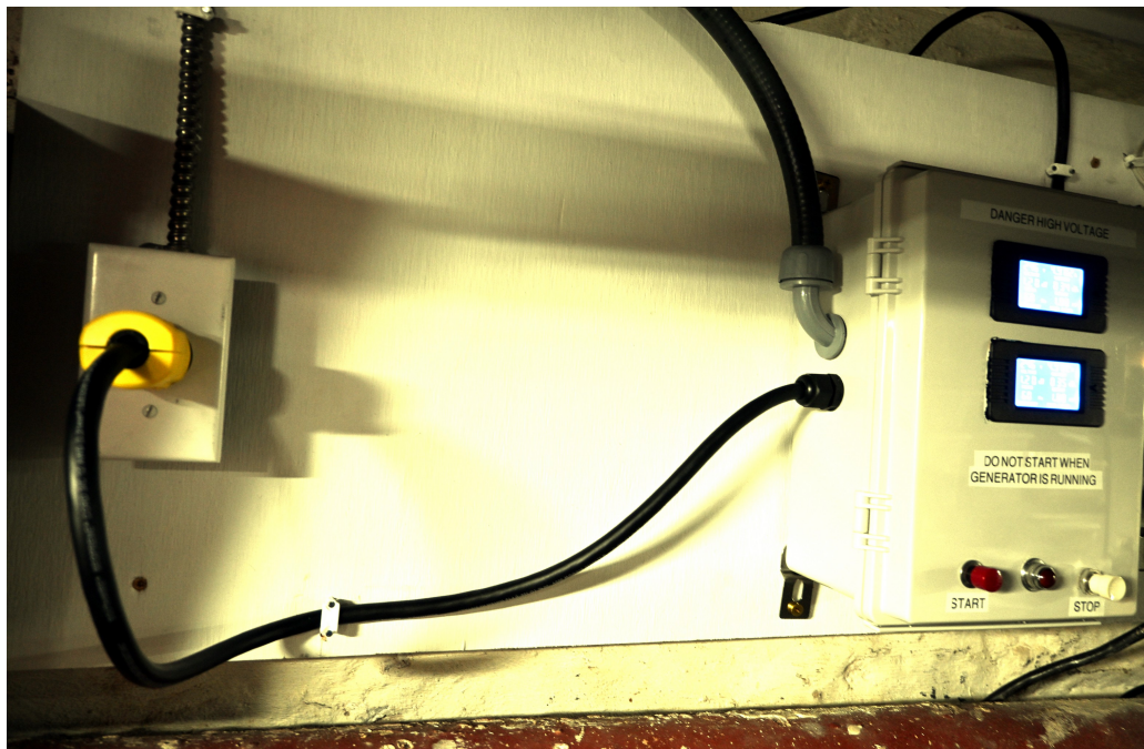
This is “plug in” solar. The output of the control box goes to a 240VAC plug and to my main panel and a 240VAC 15A double breaker.
